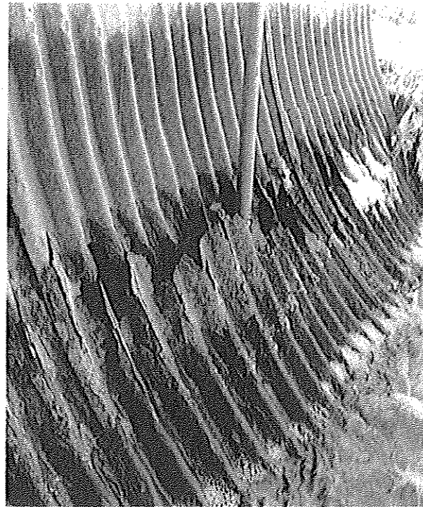
Severe corrosion with perforations and loss of fill at waterline of corrugated metal pipe.
