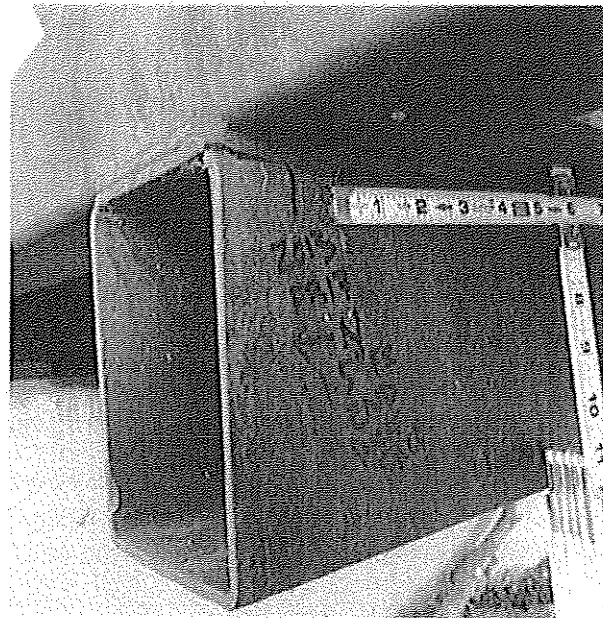
Inspection photo of cracked tubular floorbeam at welded connection of pedestrian truss.
