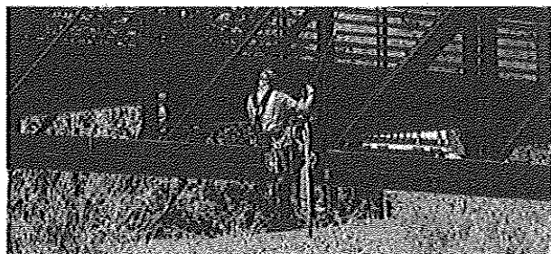
Project Manager, Adam Leith, using rope access methods to inspect pedestrian truss.
