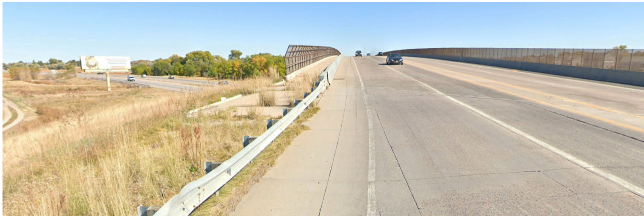
FIGURE 1. SIDEWALK OVER I-76 RESTRICTED BY GUARDRAILS AND LACKING CONNECTIVITY AT BOTH ENDS
