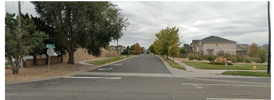
FIGURE 3. MOLINE/120TH – INCOMPLETE CURB RAMP WITH ADA COMPLIANCE ON ONE SIDE BUT NO CONNECTION TO SIDEWALK ON ADJACENT SIDE.
