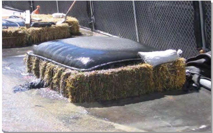
Photograph DW-1. A relatively small dewatering operation using straw bales and a dewatering bag.
