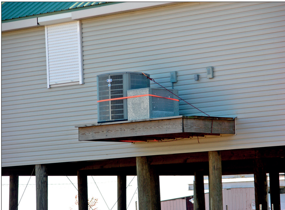
Figure 9-2. Air conditioning/ heat pump compressor mounted on a cantilevered platform attached to a home elevated on an open foundation. (Source: FEMA P-55 Figure 12-2)
