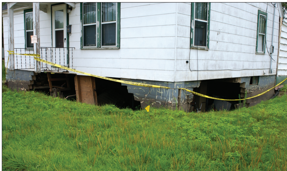
Figure 2-7. The walls of this basement in Wisconsin failed because of the pressure exerted by water and saturated soil.
