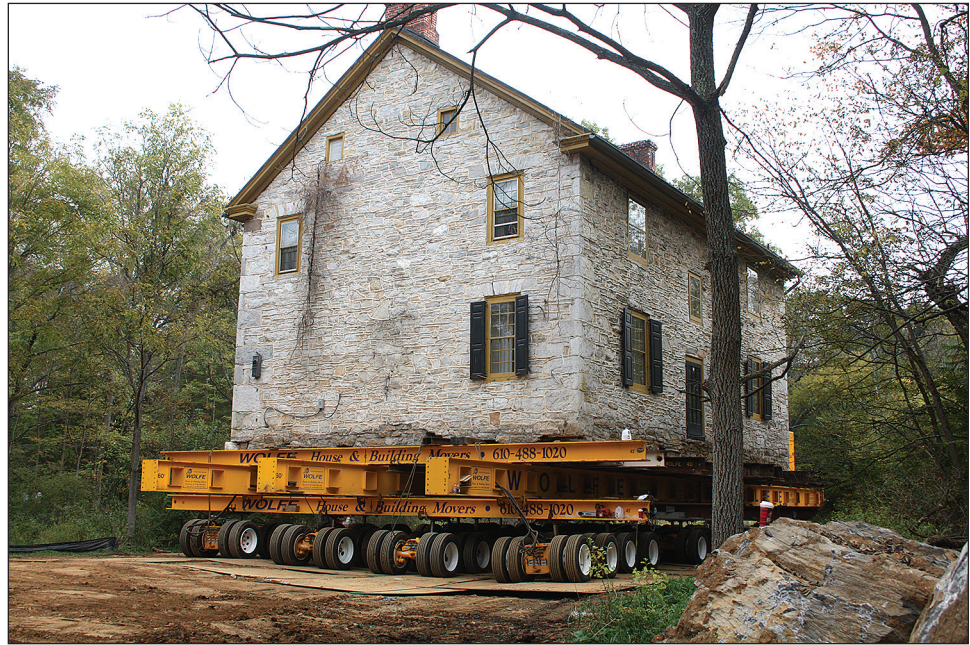
Figure 6-7. The move to the new site begins (photo courtesy of Wolfe House Movers).
