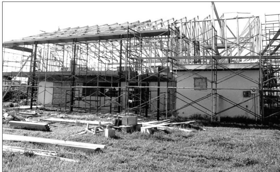
Figure 3-12. The owner of this flood-prone home in south Florida decided to build a new wood-framed second story on top of the masonry first story. The new second story is well above the BFE.
