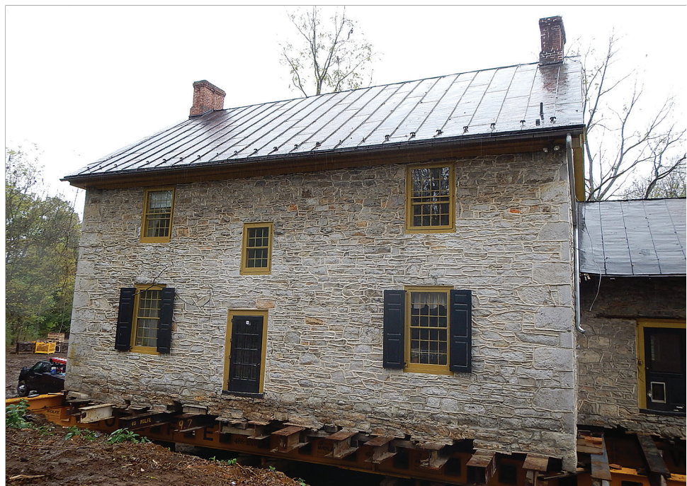
Figure 6-8. House is lowered and connected to the foundation after the foundation is fully constructed (photo courtesy of Wolfe House Movers).
