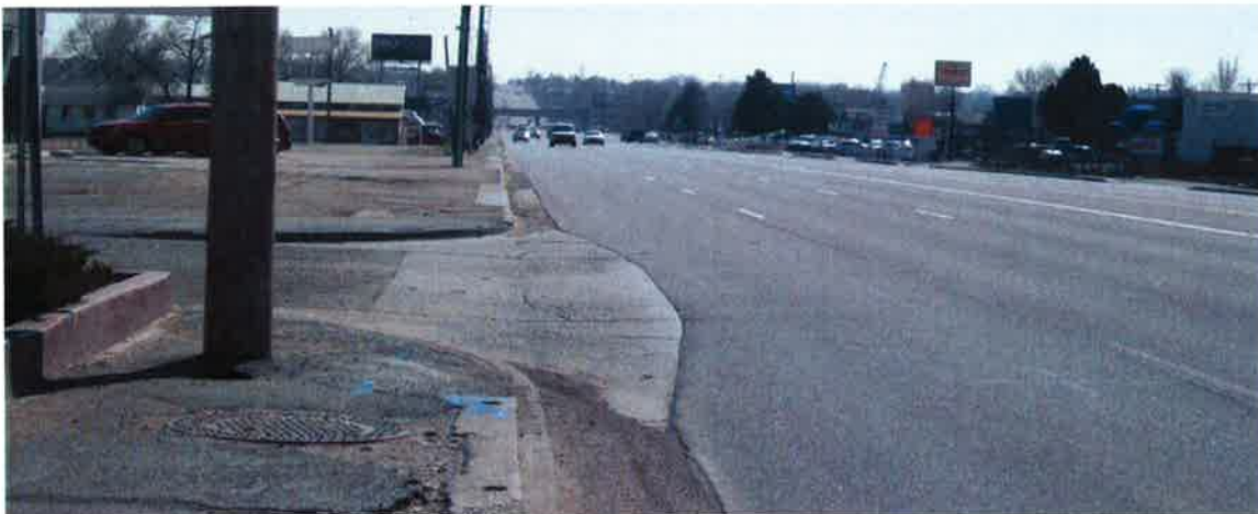
Figure 22: Many unsignalized intersections like the one shown above near 63 rd Avenue do not have ADA curb ramps or crosswalks in the Corridor
