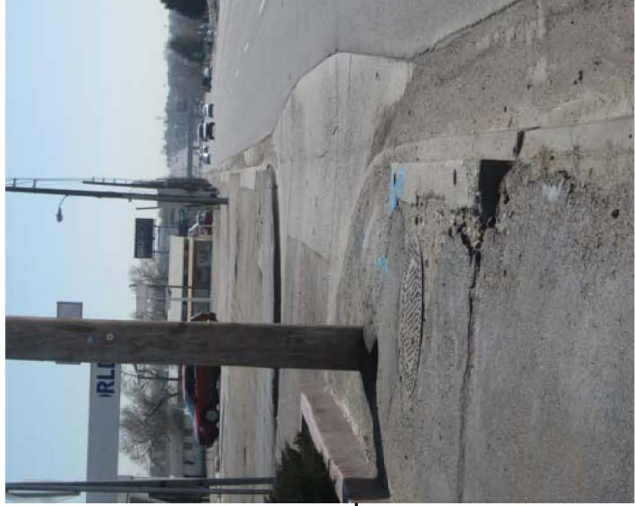
MOST UNSIGNALIZED INTERSECTIONS DO NOT HAVE A.D.A. RAMPS OR CROSSWALKS
